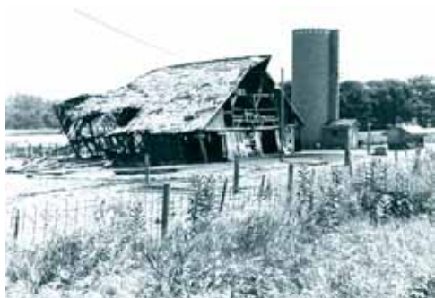
A COLLAPSING BARN AT THE JOHN COCHRAN HOMESTEAD ON THE OUTSKIRTS OF GLASGOW, IOWA, THAT HAS SINCE BEEN TORN DOWN, 1995.
